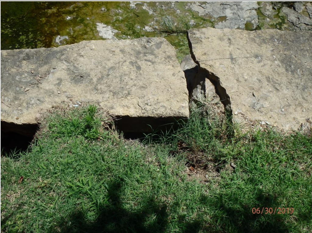
D – HOLE REPAIR - $500
