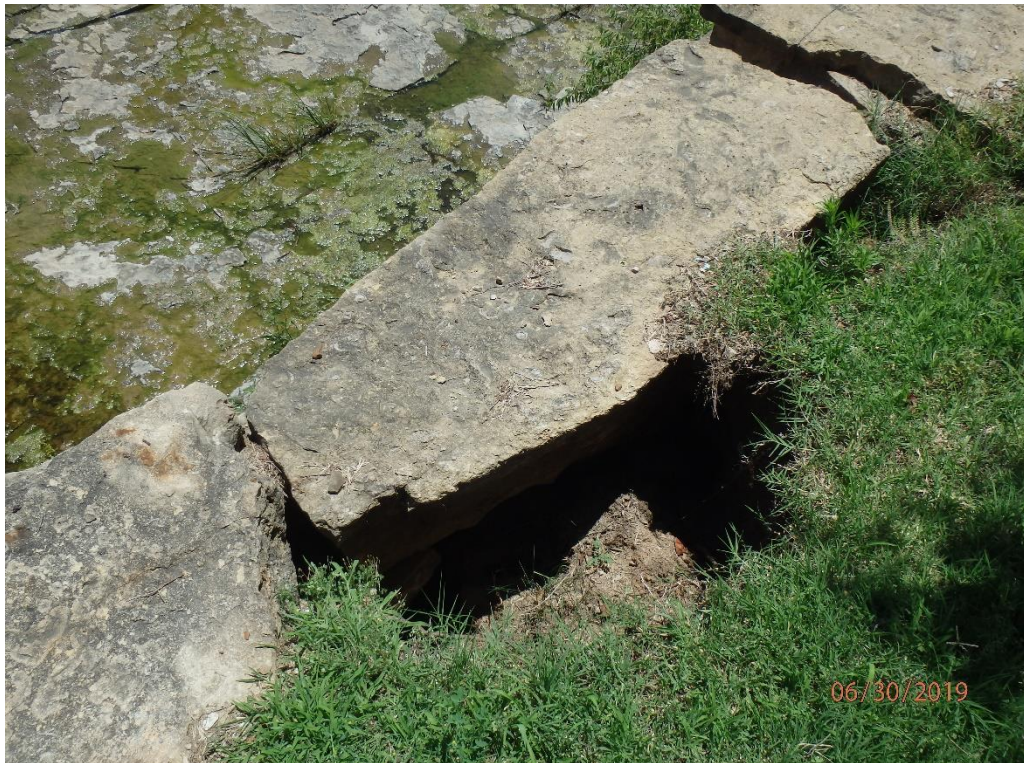
E – HOLE REPAIR - $500
