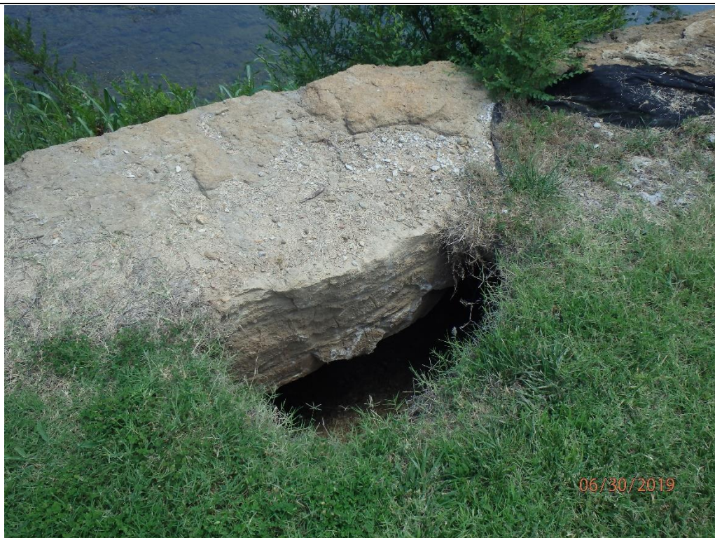
B – HOLE REPAIR - $500
